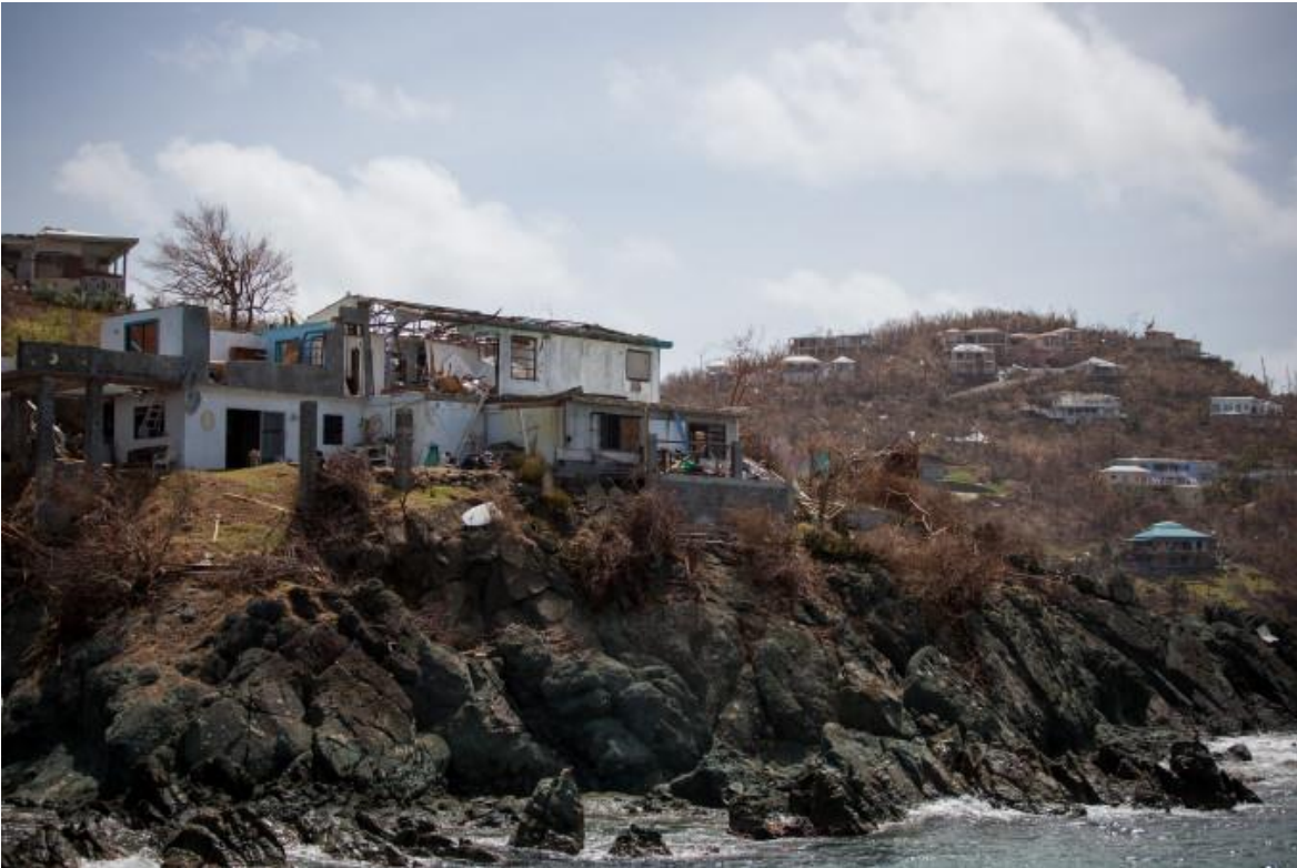
A damaged building is seen after Hurricane Irma hit St. John in the U.S. Virgin Islands. Michael Nagle/Bloomberg
